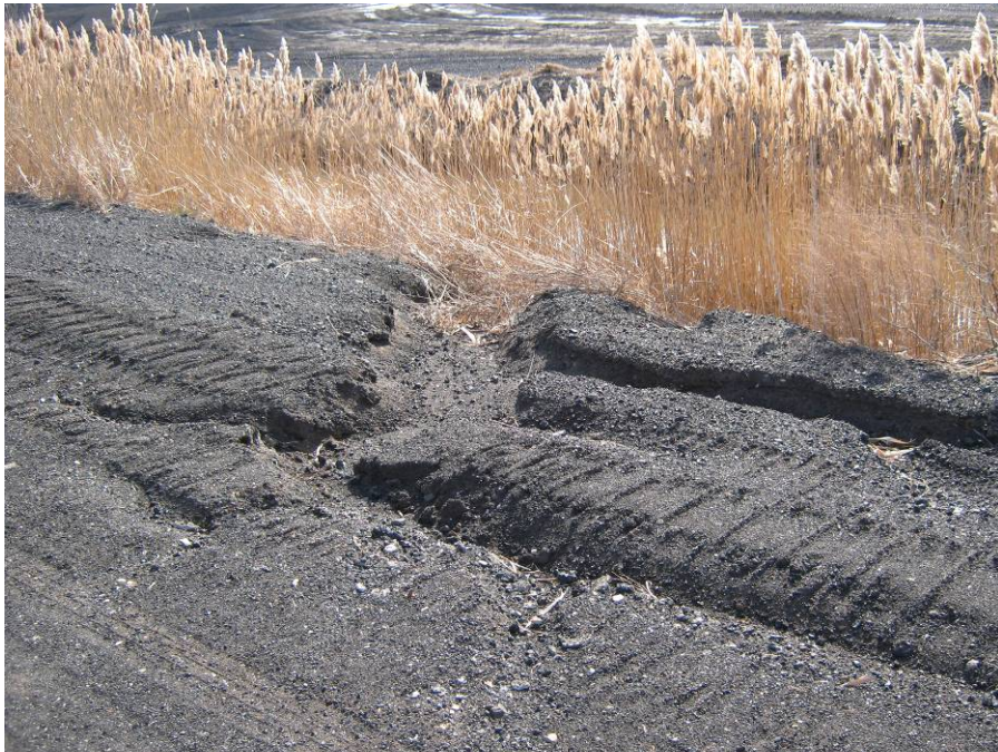
Drawing Mark AP-1-9 Erosion along divider dike between Dry Ash Stack and Ash Pond.
