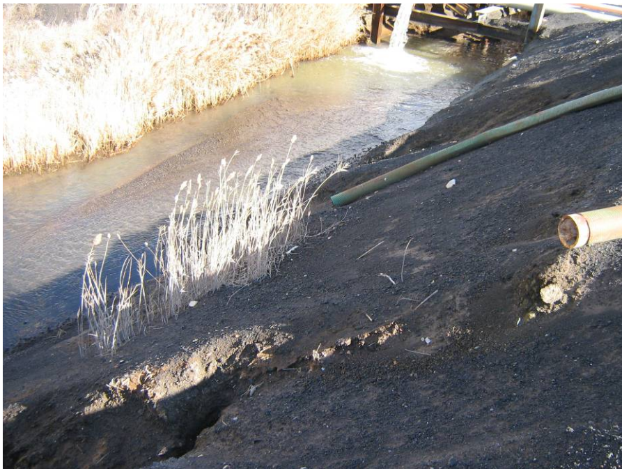
Drawing Mark AP-1-8 Erosion along north outslope of Bottom Ash Area.
