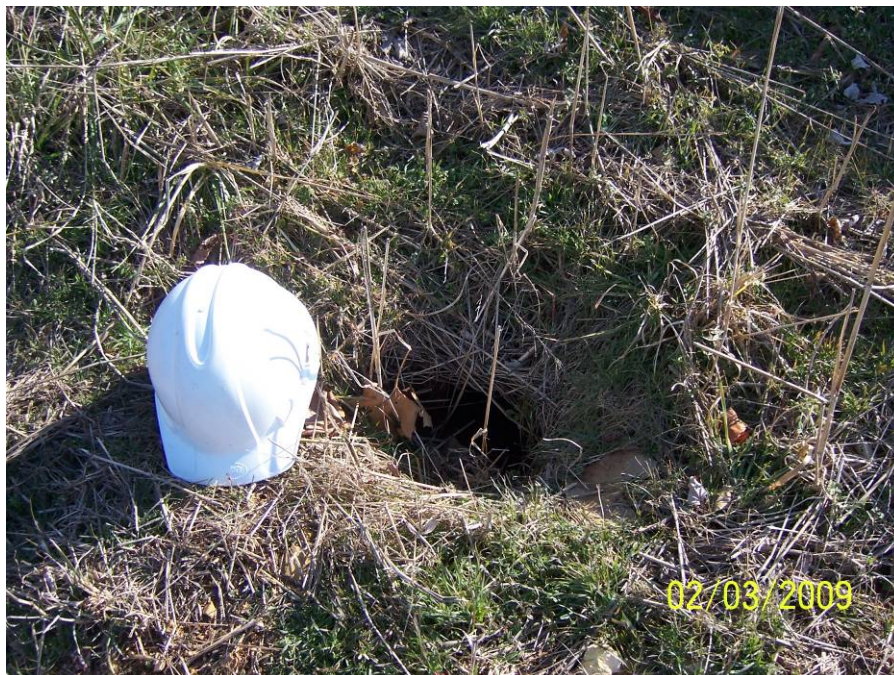
Drawing Mark AP-1-2 Animal burrow along north perimeter dike of Ash Pond.
