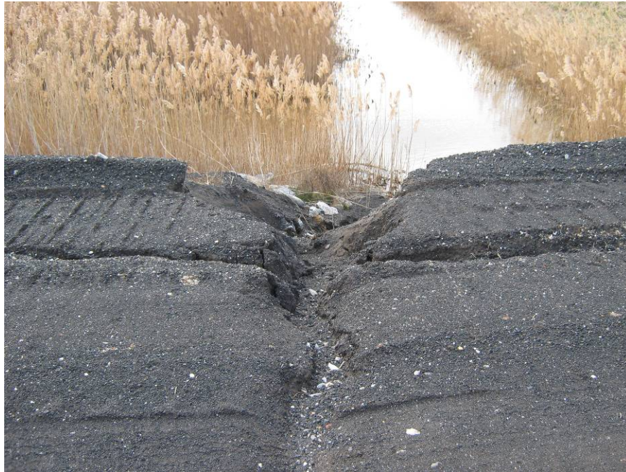
Drawing Mark AP-1-7 Erosion around 36" HDPE drain pipe along the west end of the divider dike.
