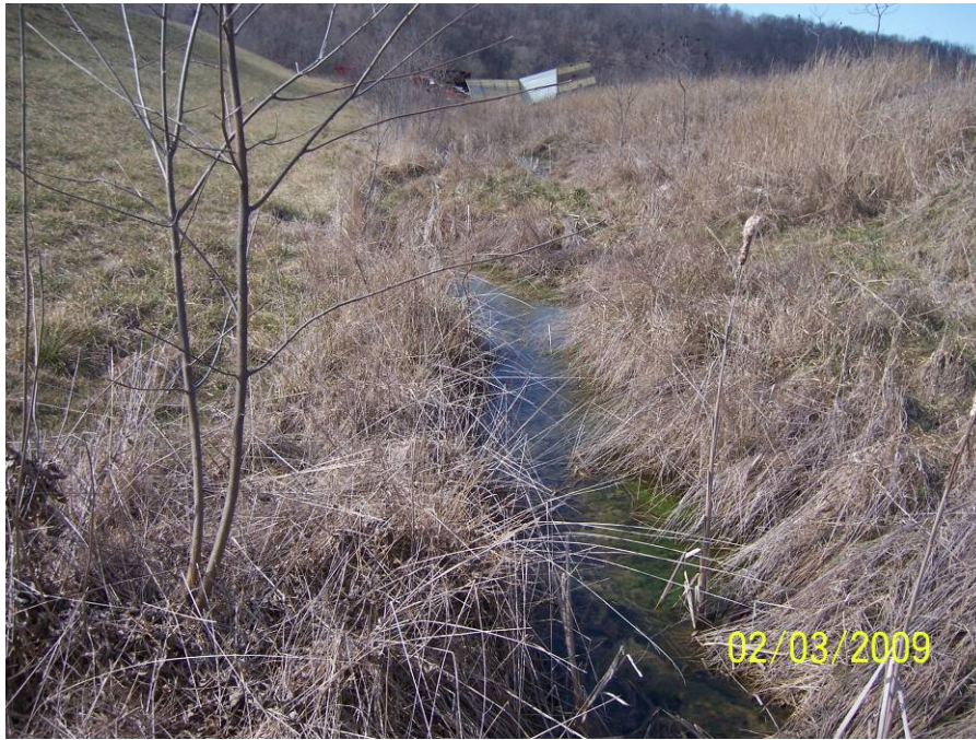
Drawing Mark AP-1-3 Standing water along toe of north perimeter Ash Pond dike.
